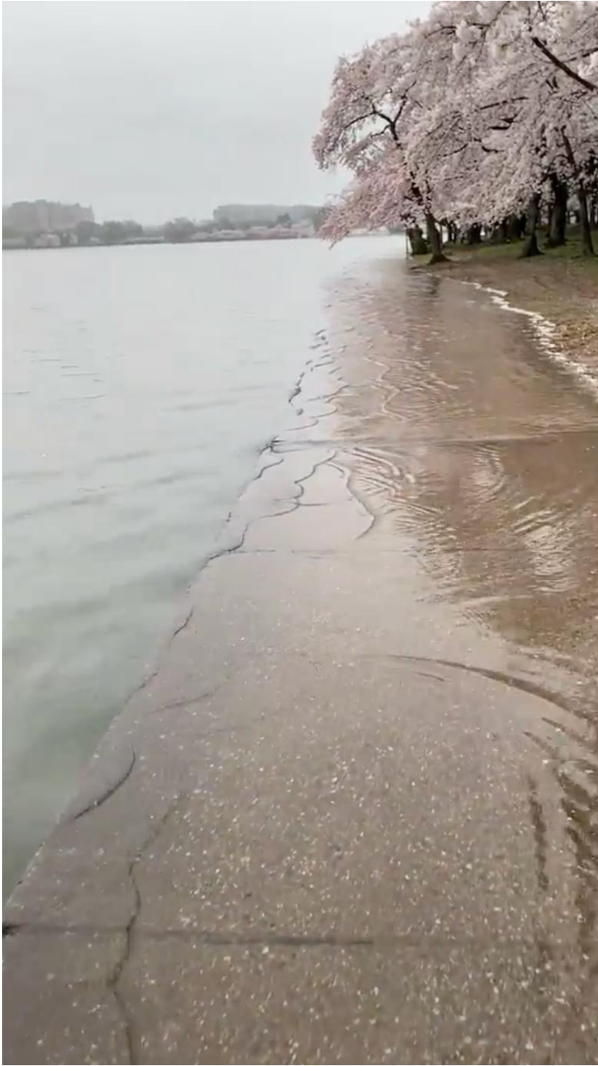
FDR Memorial seawall 3/25/2023
